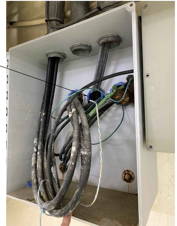
JUNCTION BOX AT MAIN PUMP BUILDING
