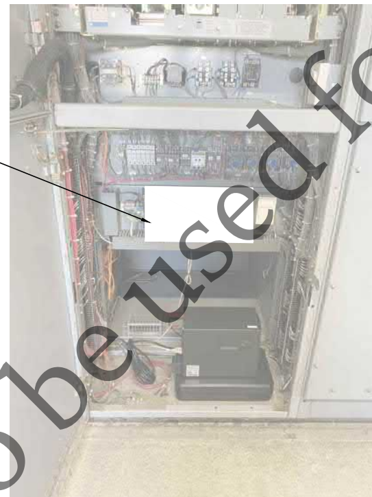
MAIN SWITCHGEAR CONTROL CUBICLE MAIN SWITCHGEAR BUILDING
