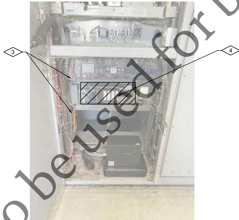
MAIN SWITCHGEAR PLC AND CONTROL CUBICLE - REMOVAL MAIN SWITCHGEAR BUILDING
